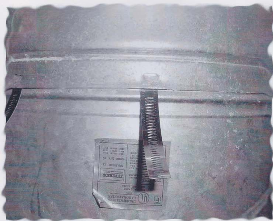
Using a flat head screwdriver to gently pry open twist lock pipe joints so steel shims can be inserted.
