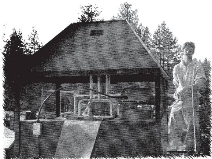
Neal Hooper takes a break from sanding and painting the damaged chimney cap.
