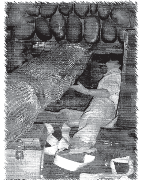
Neal Hooper observes the liner's progress as it is winched up the chimney.
